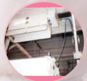
Autoregulator Connected With Autofeeder Over Gin Machine With Sensor
